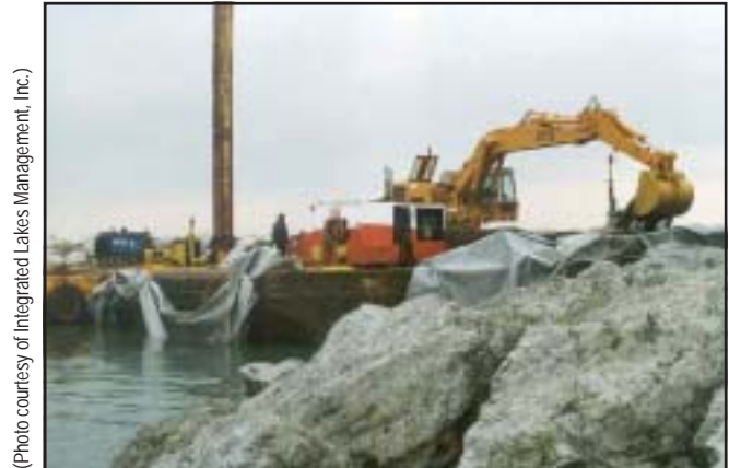
Dredging is an eventual cost. Plan ahead and set funds aside.
